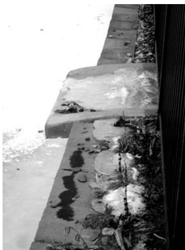
Figure 5-12. Example MSE wall overflow sill at top of wall.
