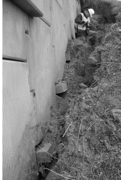
Figure 5-16. Example of surface flow erosion at the bottom of an MSE wall.
